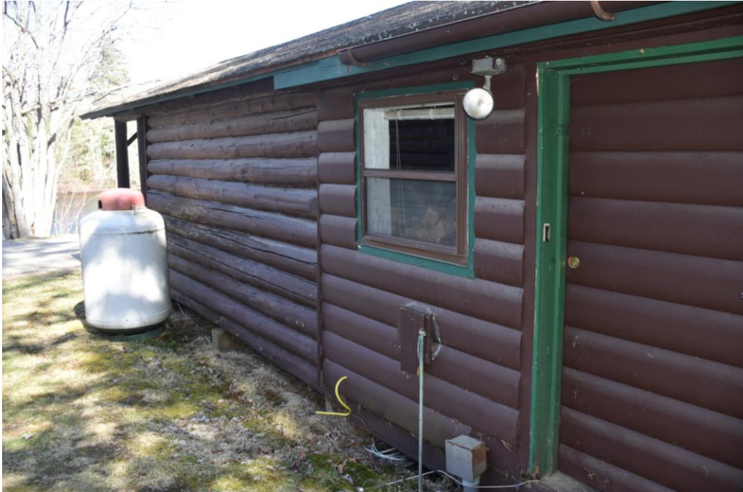
Photo 10) Manager's cabin north elevation showing 1970s back addition Reference (file name): PIC_2490
